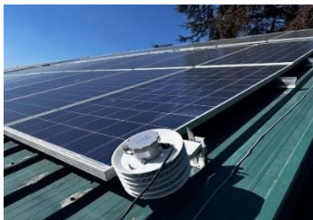
Figure.8: Ambient temperature sensor
