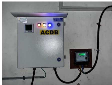
Figure 5: AC distribution box
