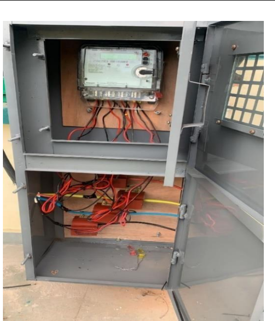
Figure 6: Power Generation meter
