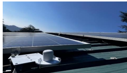
Figure.9: Solar radiation sensor
